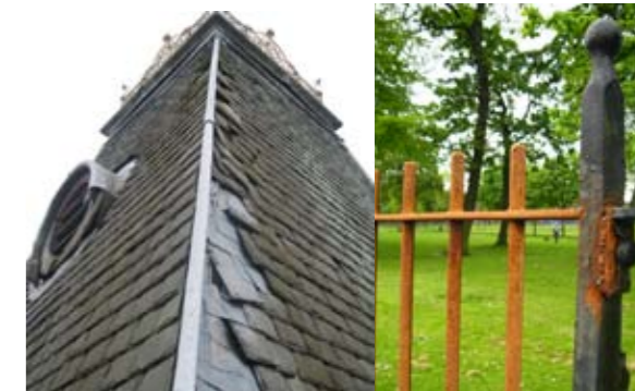
Missing slates at Water Row & rusted railings at Elder Park
