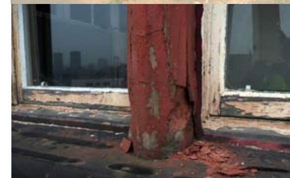
Above: Flaking paintwork on windows at Water Row
